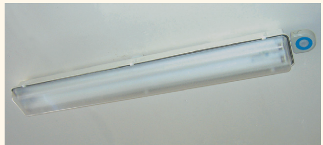
FIGURE 1: BI-LEVEL FLUORESCENT PARKING GARAGE LUMINAIRE Parking Garage 22, University of California, Santa Barbara
