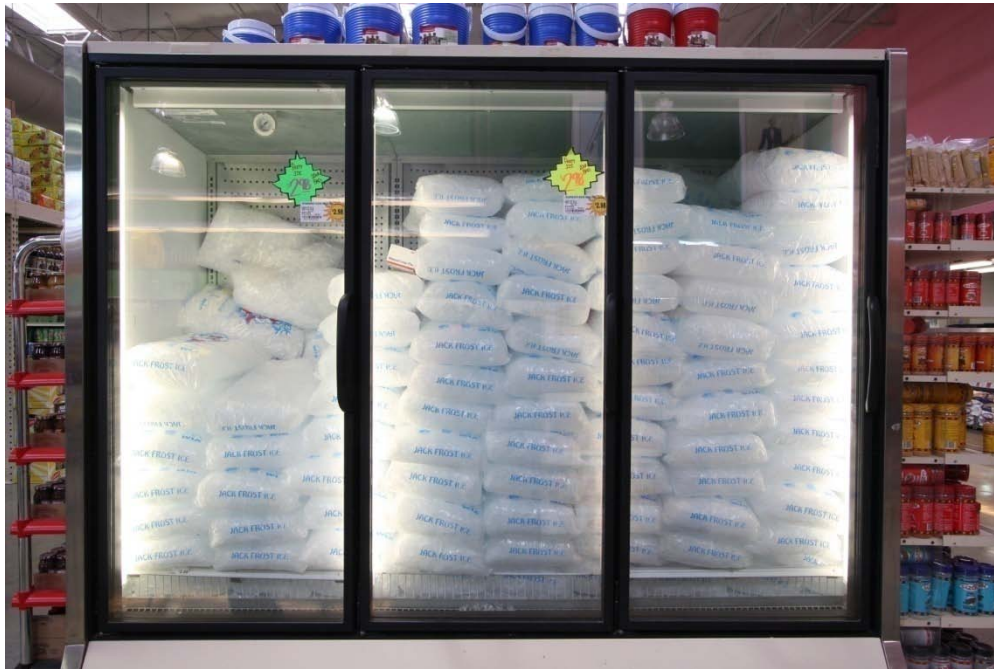
Figure 4-1 Baseline Lighting (T8 Fluorescent Lamps)
