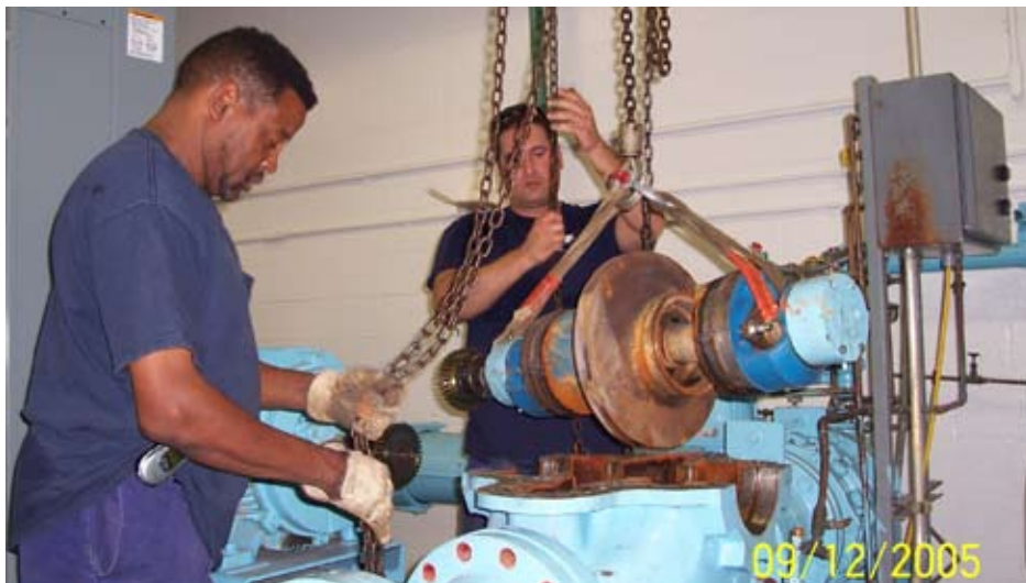
Figure 1. Denise No. 2 horizontal split-case pump being taken out of service for repair and coating.
