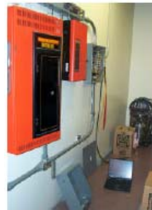
Figure 5.2.4-1: The Envenergy installation
