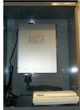
Figure 5.2.4-2: The Envenergy controller
