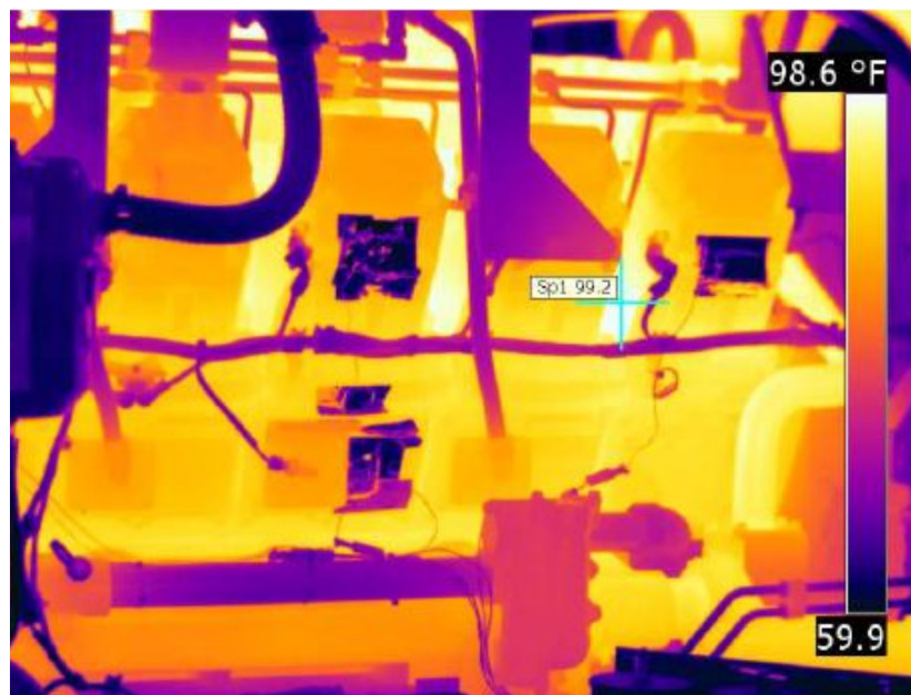
FIGURE 18. ENGINE GENERATOR #2 (FC EGBH) – TOP #3
