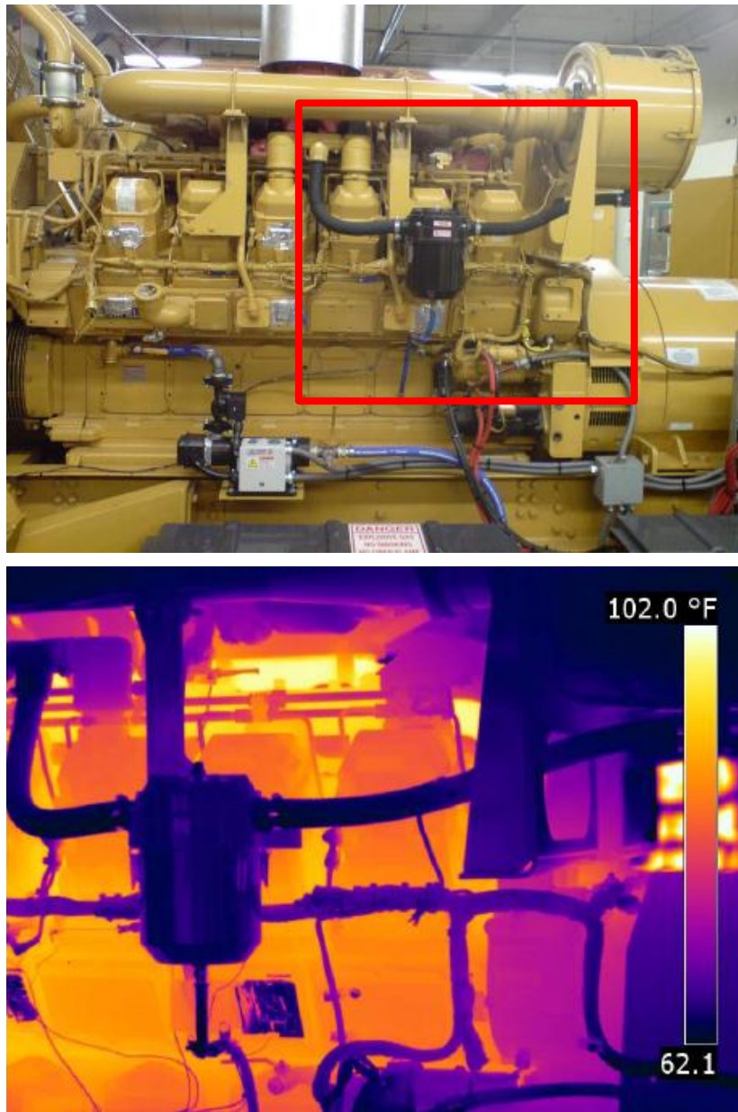
FIGURE 17. ENGINE GENERATOR #2 (FC EGBH) – TOP #2
