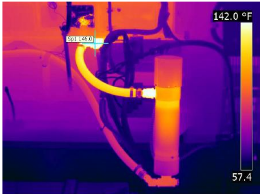
FIGURE 20. ENGINE GENERATOR #3 (TS EGBH) – TS HEATER CLOSEUP/SUPPLY LINE
