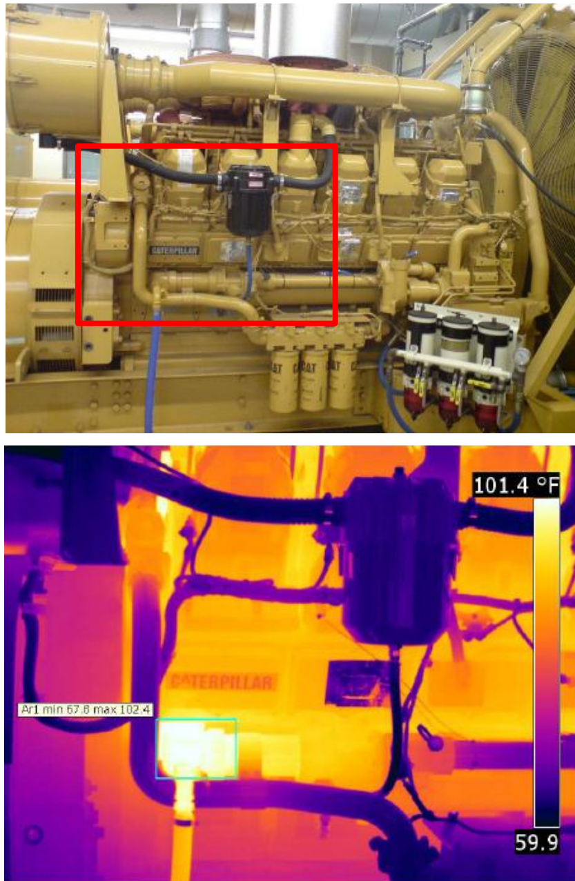
FIGURE 19. ENGINE GENERATOR #2 (FC EGBH) – FC EGBH RETURN LINE
