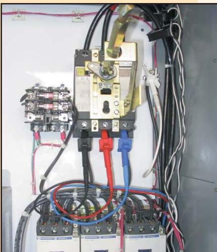
Probes measure amperage in one of three variable speed drive units for the kitchen hood fans.
