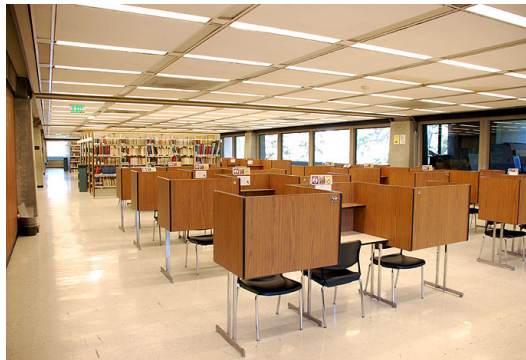
The Moffitt Library lighting retrofit saves over 3 kWh per square foot per year. Photo: Charlie Huizenga.
