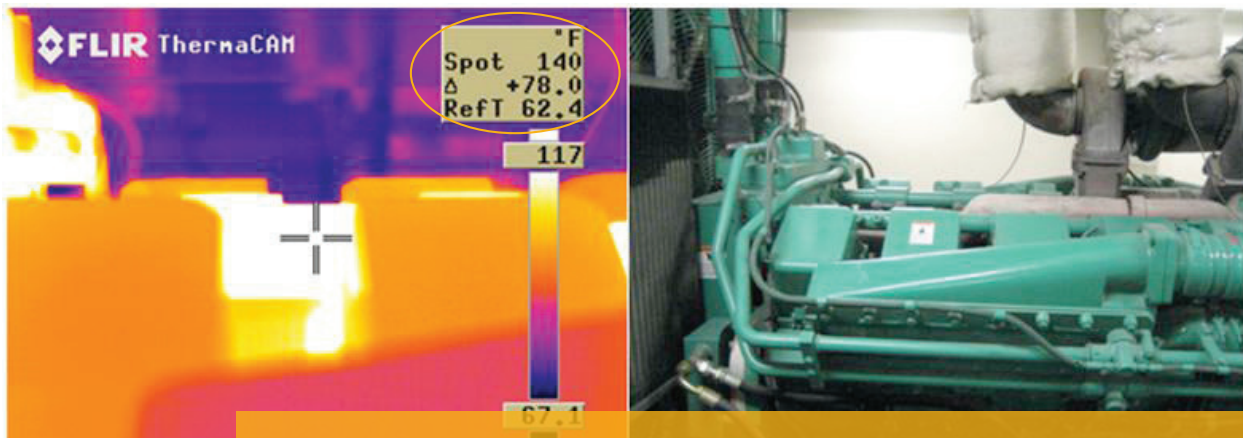
Figure 3: Generator A thermosiphon, thermal and normal image of top of engine, spot temperature 140°F
