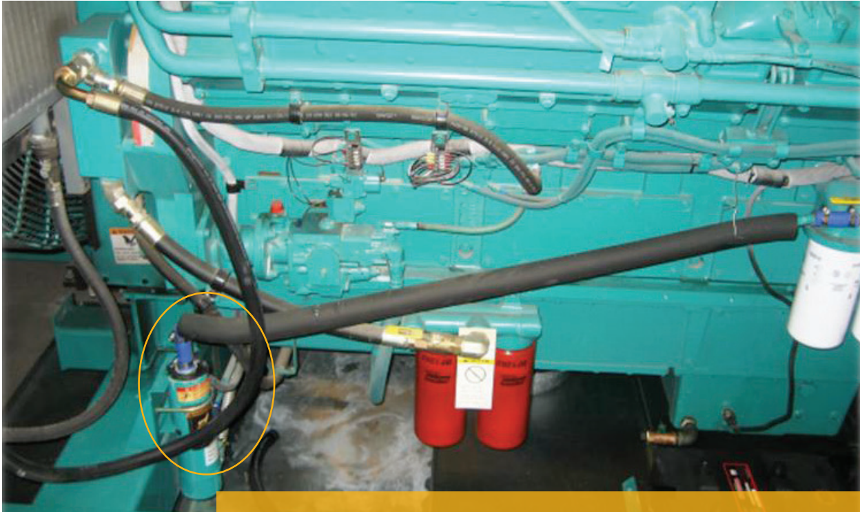
Figure 1: Example of thermosiphon engine block heater as installed on a typical standby generator.
